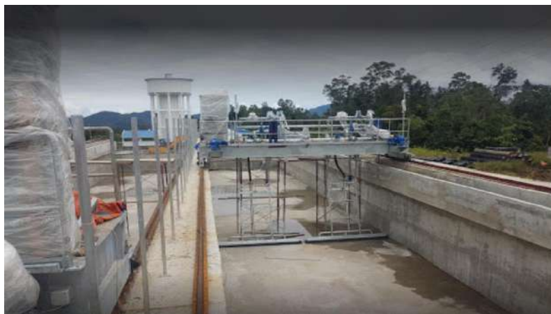
Figure 4-13: Bayai Water Treatment Plant
