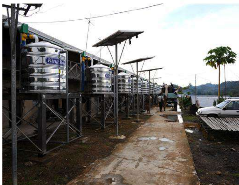
Figure 4-14: Rainwater Harvesting System at Bair Longhouse, Betong
